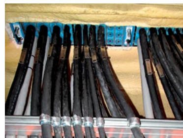
Fig. 7 Correct cable sealing with Roxtec
