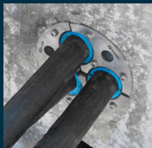
Cable draw pit
