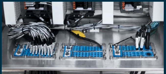
Surveillance and IoT cabinets
